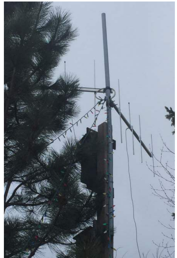
THE FIXED RADIO-TELEMETRY STATION JUST DOWNSTREAM OF THE BURRARD BRIDGE IN VANDERHOOF. WHENEVER A STURGEON WITH A RADIO-TRANSMITTER PASSES BY THIS ANTENNAE, THE DATE AND TIME ARE RECORDED. PHOTO COURTESY WAYNE SALEWSKI.
