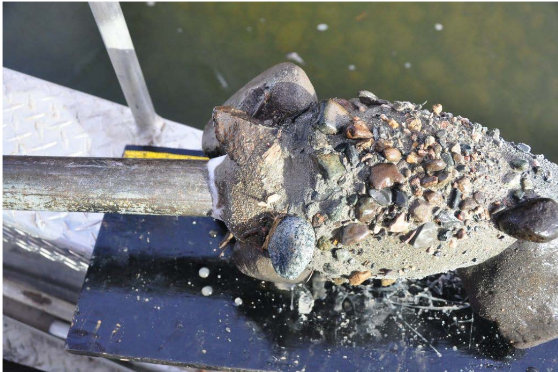
Photo 67: Core 18 (Lower Patch)
